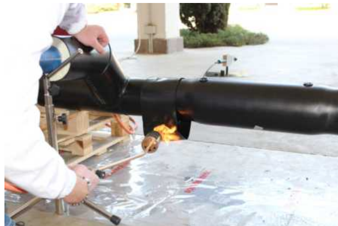
16 - Perform the welding operation, heat the band by using the torch in all directions until it has completely shrunk. Repeat the operation for both bands.
